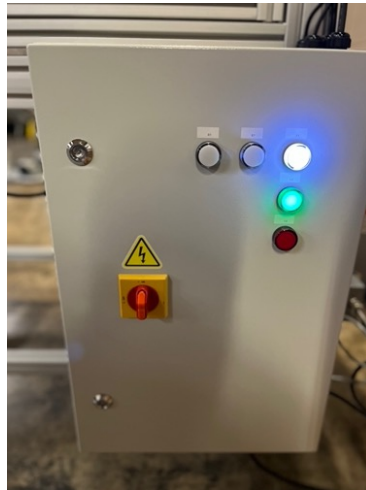
Main electrical cabinet with Power and "ready" indicator lights.
