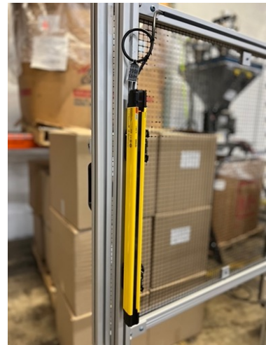
Light curtain mounted to access door / interlock.
